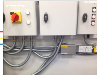
415 V AC Microgrid
