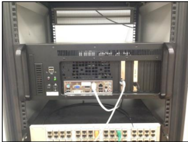
AC/AC Converter RT Controller
